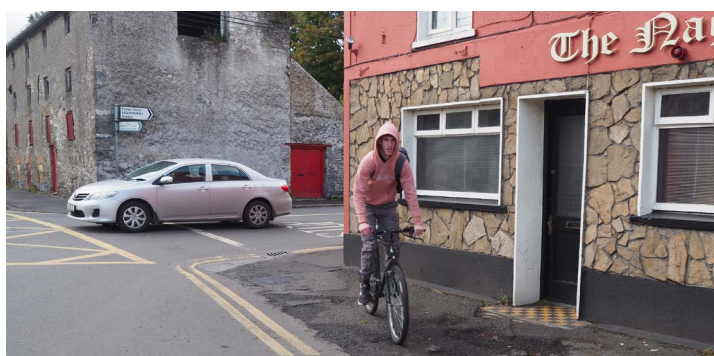
E Degraded kerb conditions and delineations create ambiguity between different travel modes.
